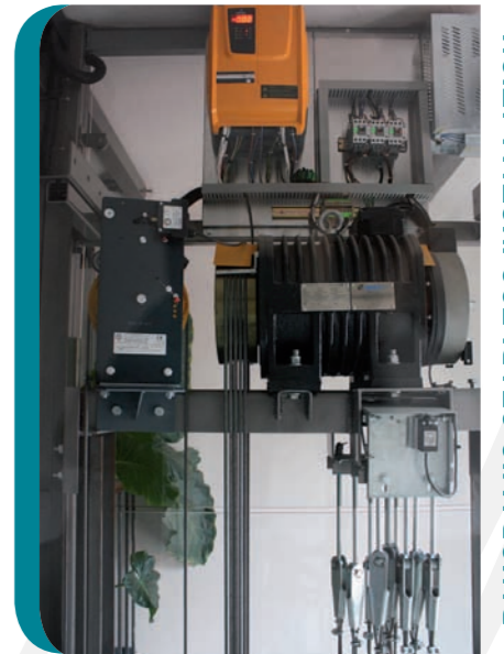
PANORAMIC GEARLESS INSTALLATION
